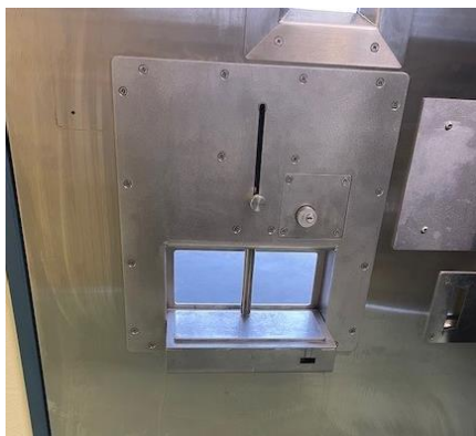
A drop pin installed in a prison cell door
